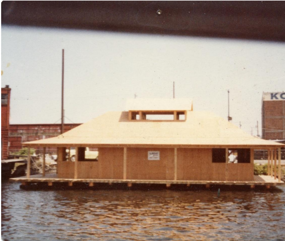
B18. Boat Shop under construction, 1982 or 1983. Source: Center for Wooden Boats collection.
